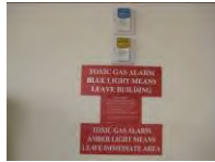
5.10 Toxic Gas Alarm Enunciator and Strobe
